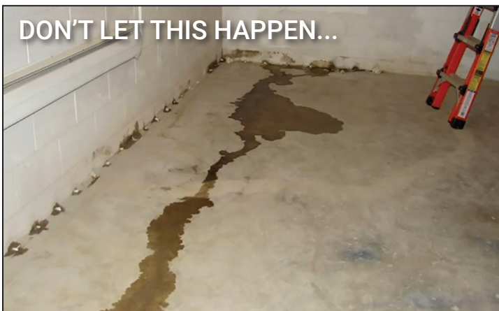
A waterproofing job where PolyCove wasn't used and the concrete replacement floor blocked the weep holes in the wall.
